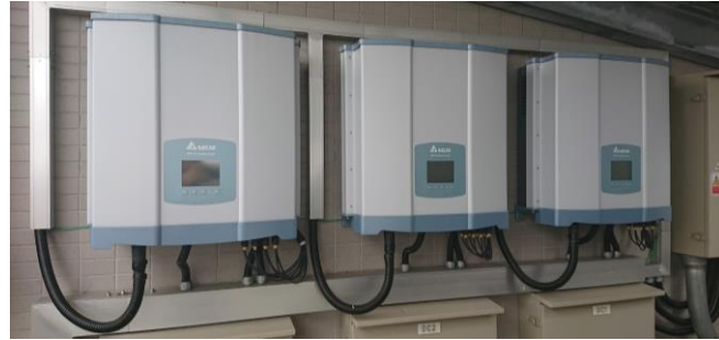
PV Inverter 1 PV Inverter 2 PV Inverter 3
