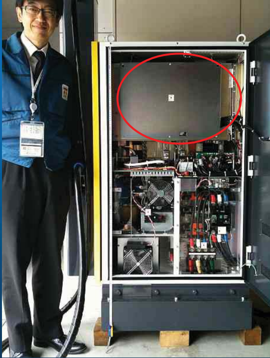
DC Off board Charger
