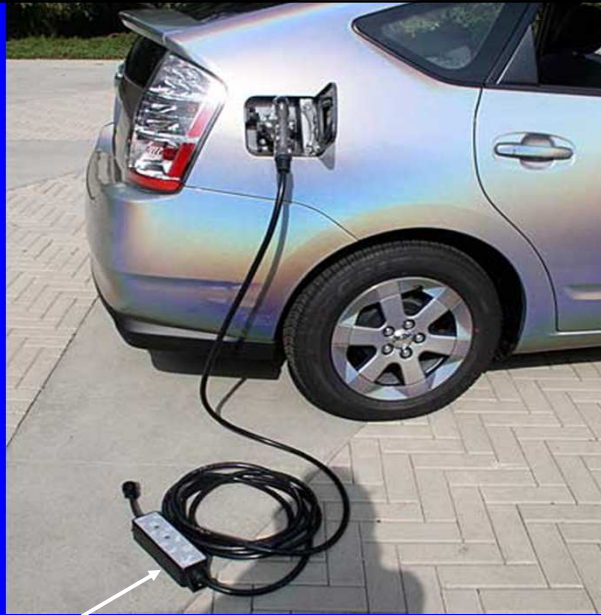
Personnel Protection system
